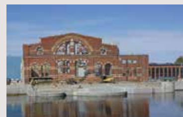
In Varvstaden in Malmö the iconic building Gjuteriet, where parts for ships were previously cast, is being turned into a modern and sustainable meeting place. The project will be completed in 2023 through Centur, a company jointly owned with Balder.
